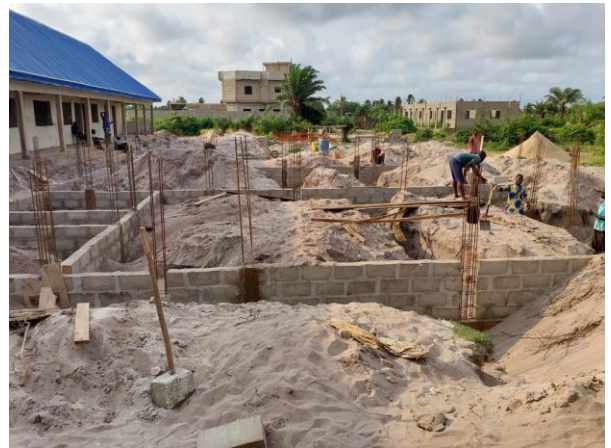
Second Stage - Laying of Foundation for the 2 story building containing 12 Classrooms and 12 Offices
